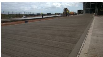
Large areas can be poured without having to negotiate in-situ steel mesh
